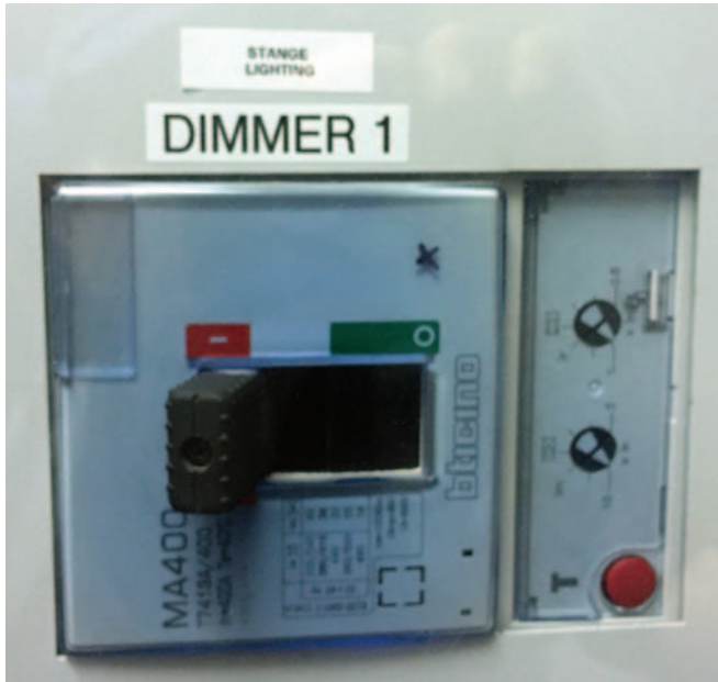
Main breaker for one of the venue's 96-dimming racks.
