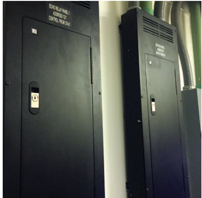
Relay panels to control non-dimmable loads at the venue.
